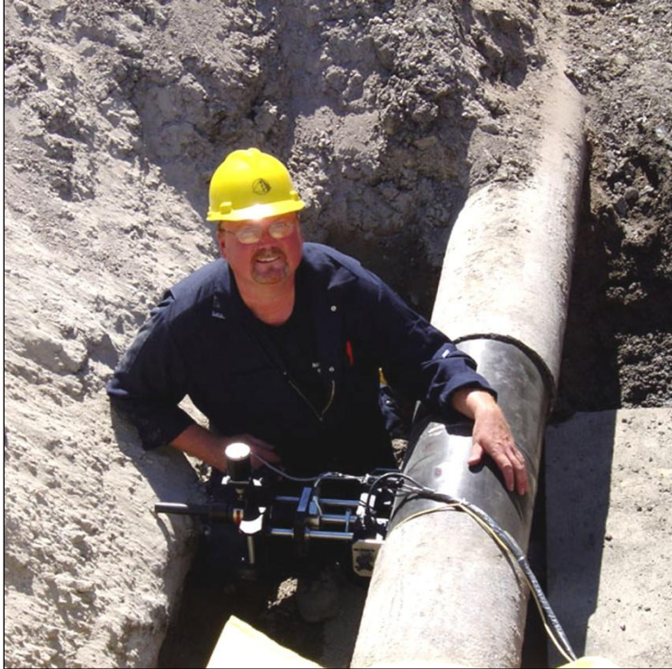
Fig. 1a In-Situ SSM system being used to test base metal of undocumented gas pipeline in order to determine its Grade. The DC electric magnets have excellent performance even at the toughest 3 O'clock and 9 O'clock positions.
